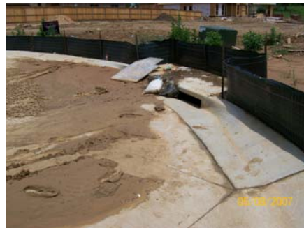
EXAMPLE OF POOR EROSION CONTROL
