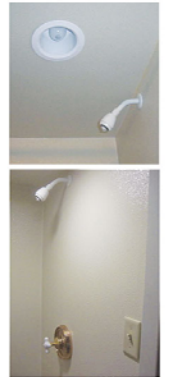
IMPROPER ELECTRICAL INSTALLATION
