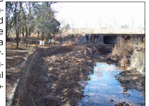
STORM WATER ISSUE
