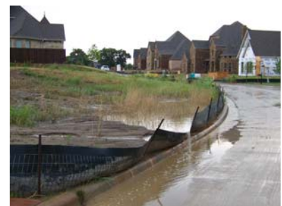
FAILED EROSION CONTROL
